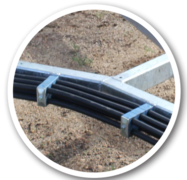
All Hydraulic Hoses Clamped In Saddles- Not zip tied
